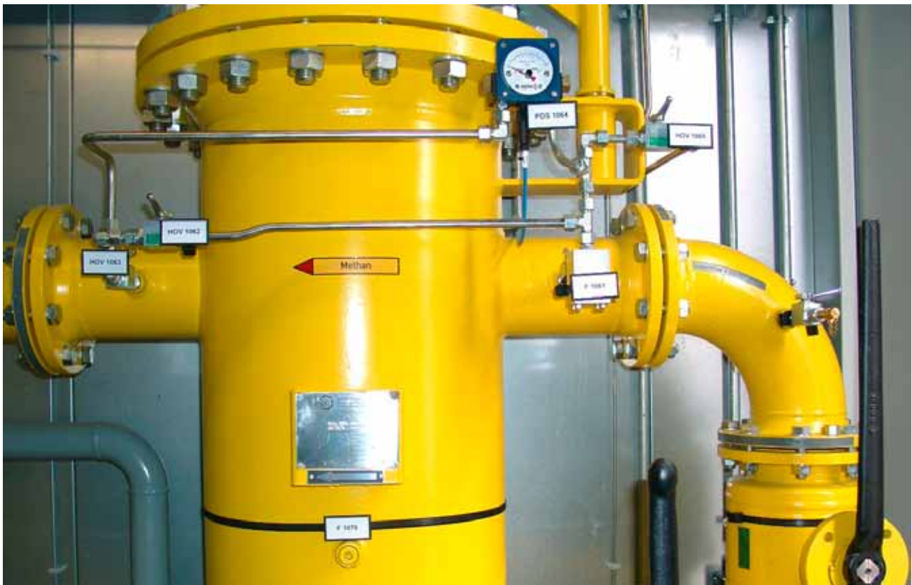
Figure 7: Biomethane piping and measurement equipment in the grid connection station
